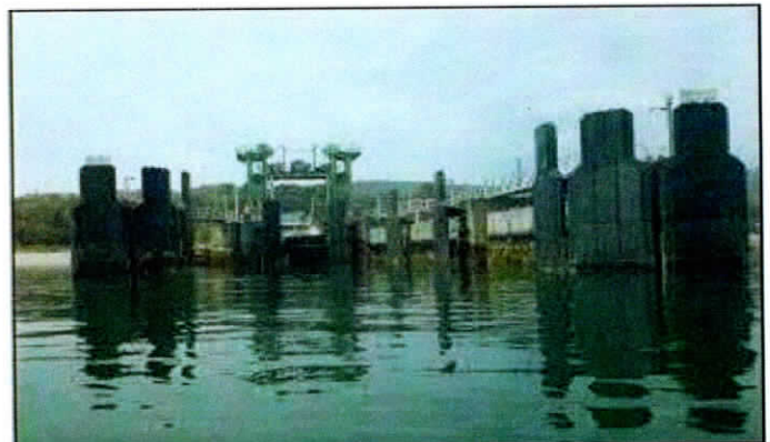
"Dolphins" with fenders at the Lincolntonville terminal.
