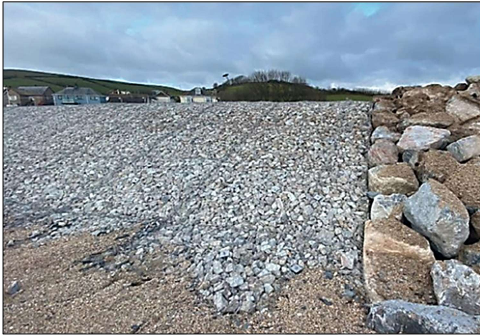
Photograph 6: Geobruigg's TECCO® CELL System Installed Beside a Traditional Rock Revetment (Photograph curtesy of Geobruigg).
